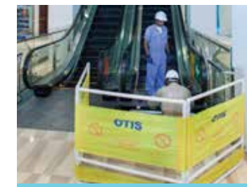
ELEVATOR / ESCALATOR / TRAV-O-LATOR MAINTENANCE
