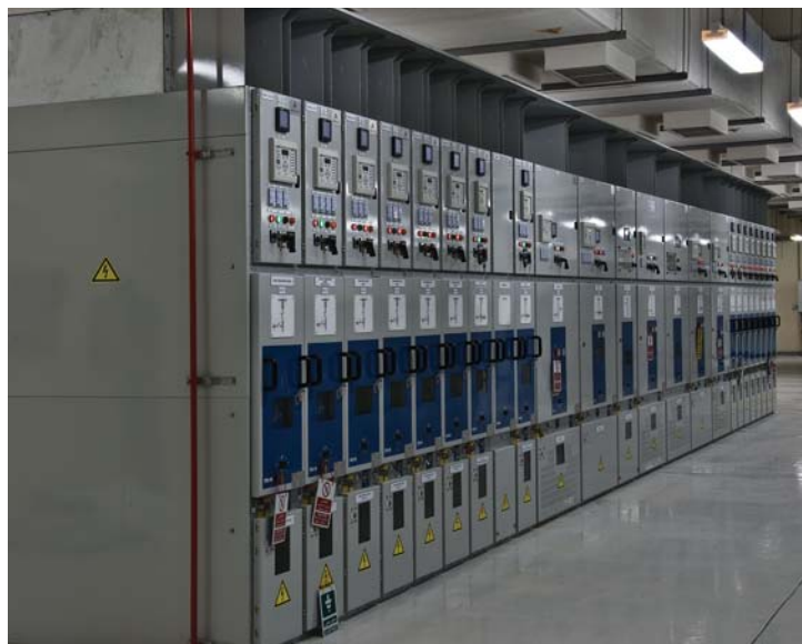
M. V. Switch Board - 6.6 kV
