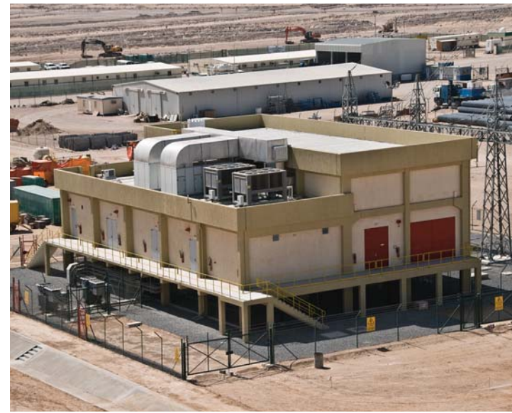
132 kV GIS Substation
