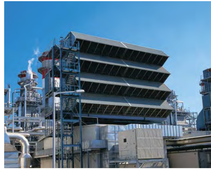
Air Intake Filter Housing of a Unit
