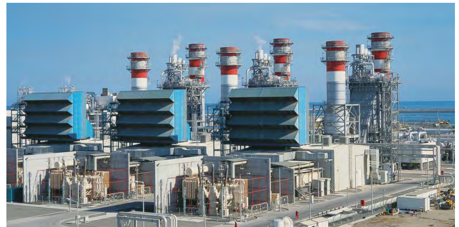
The Power and Steam Generation Units
