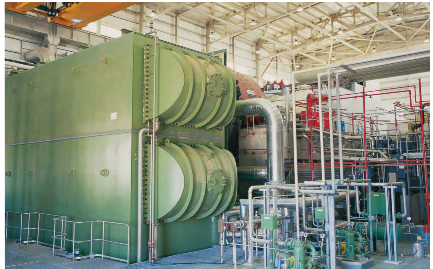
Unit around the Condenser of the Steam Turbine
