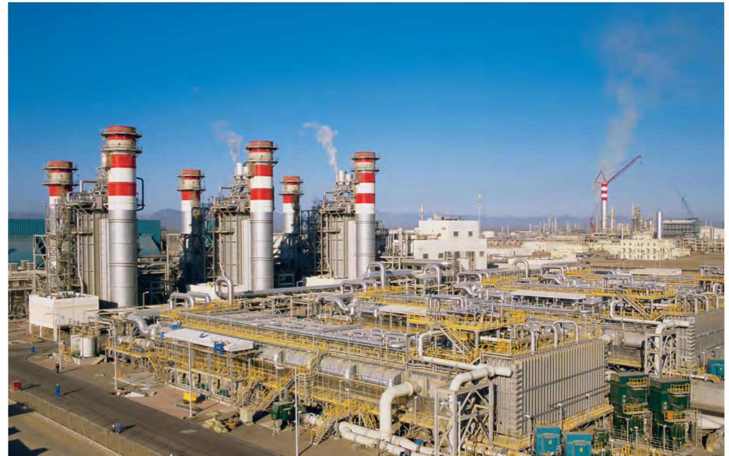
Project Management, Supervision and Mechanical, Electrical & Instrumentation Installation of the IWPP – Sohar.
