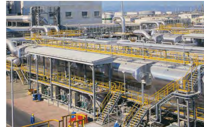
Closer view of a Desal Unit
