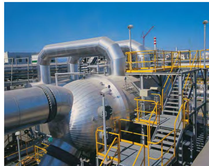
Piping around the Desal Unit
