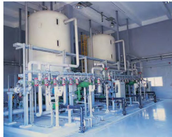
DM Water Plant
