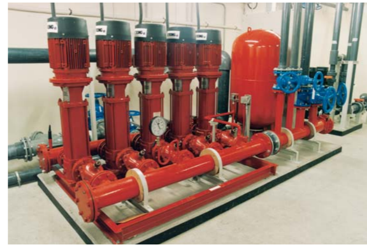
Potable Water Pumps
