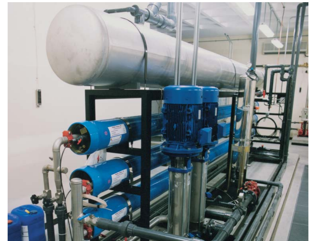
Reverse Osmosis Plant
