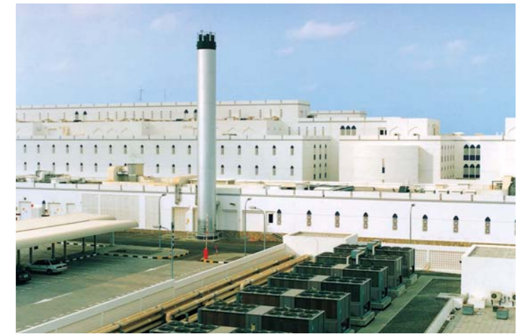
9 nos. Air Cooled Chillers
