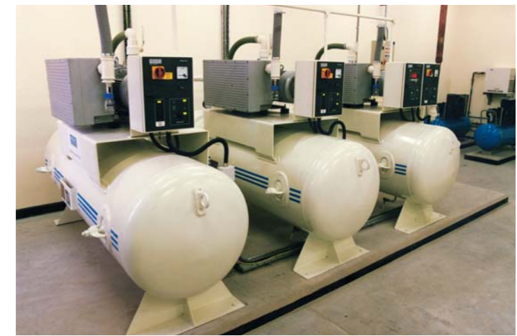
Medical Air Compressors
