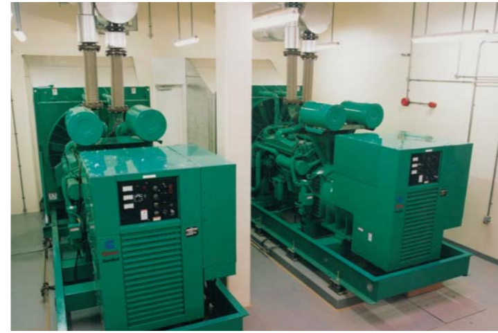
Standby Diesel Generators
