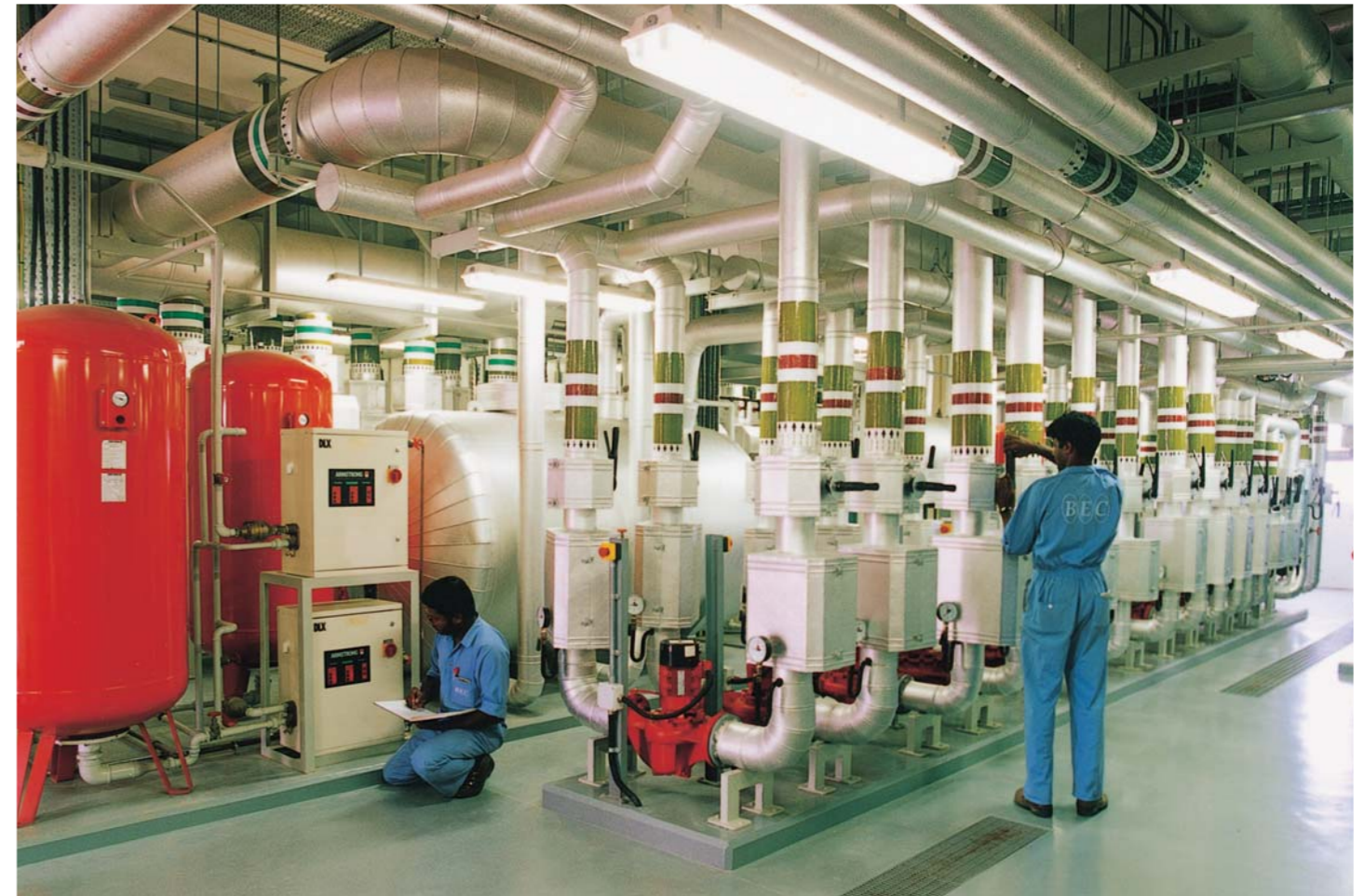
Piping in Mechanical Plant Room
