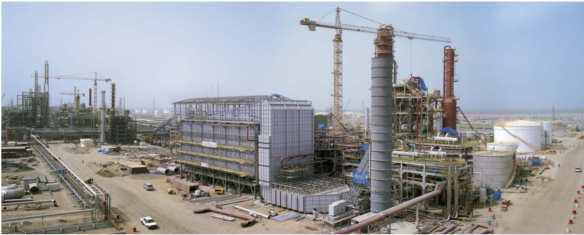
Overview of Reformer
