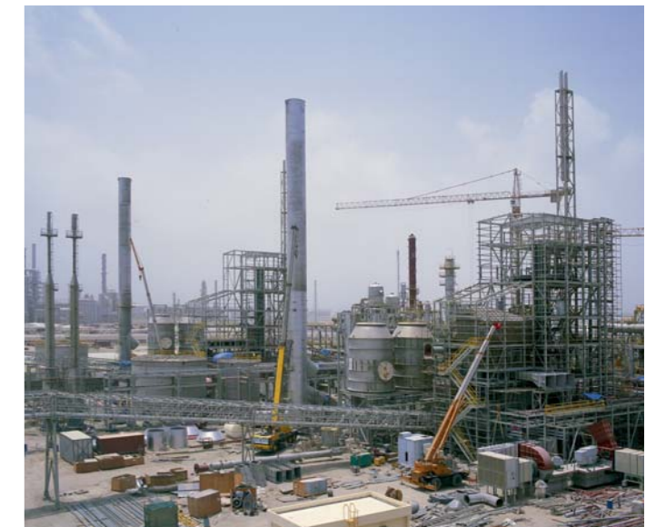
Granulation Structure & Urea Conveyor
