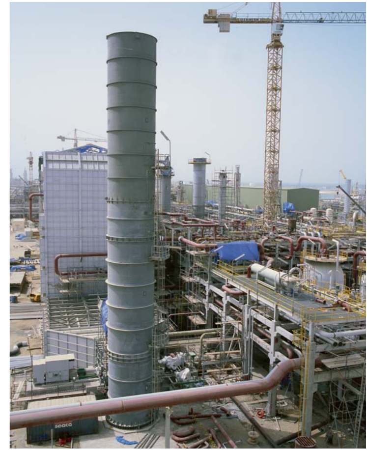
Ammonia Rack Piping
