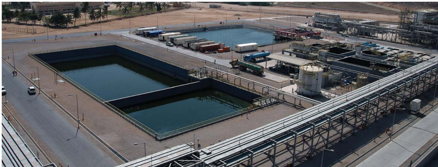
Storm Water and Fire Water Sump
