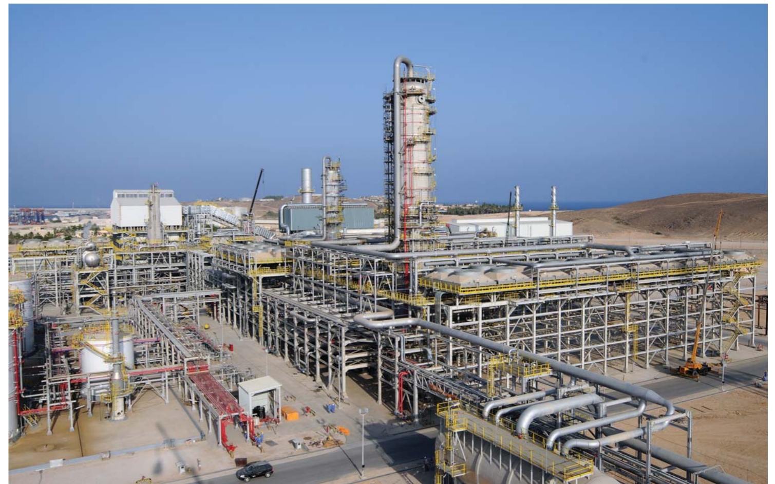
Process Area – View from Knockout Drum
