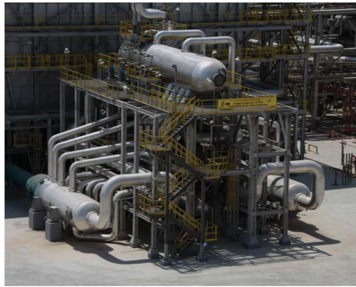
Reformer – Makeup Gas Boilers and Steam Drum
