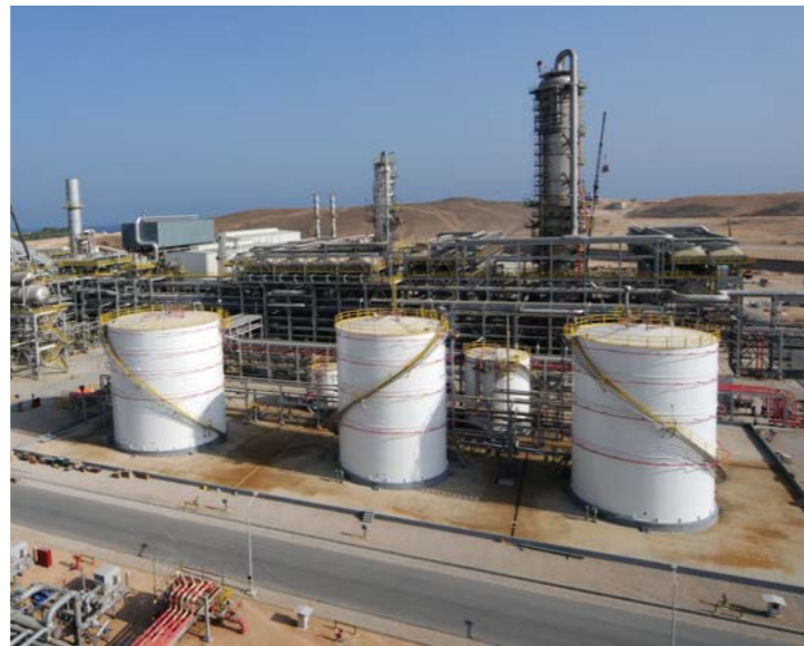
Process Storage Tanks
