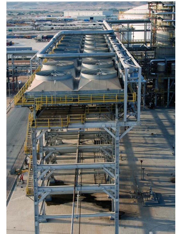
Air Coolers on Pipe Racks
