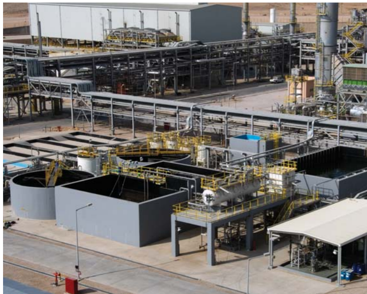
Effluent Treatment Plant
