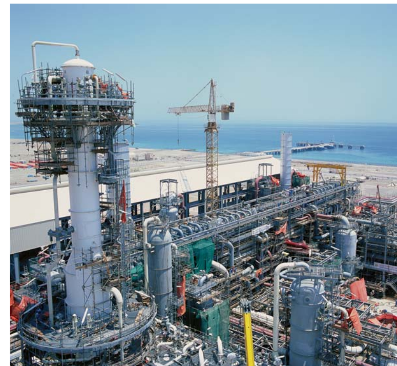
Bottom Right: Pipe Rack and Main Cryogenic Heat Exchanger.
