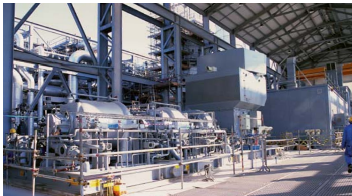
Top: View of the Process Train. Centre Left: The Two Frame 6 Gas Turbines. Centre Right: View of Compressor Shelter and Pipe Rack. Bottom: View of MR/PR Compressors.
