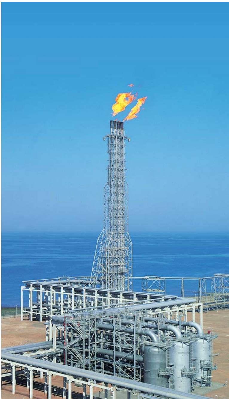
100 metres & 60 metres Flare Stack
