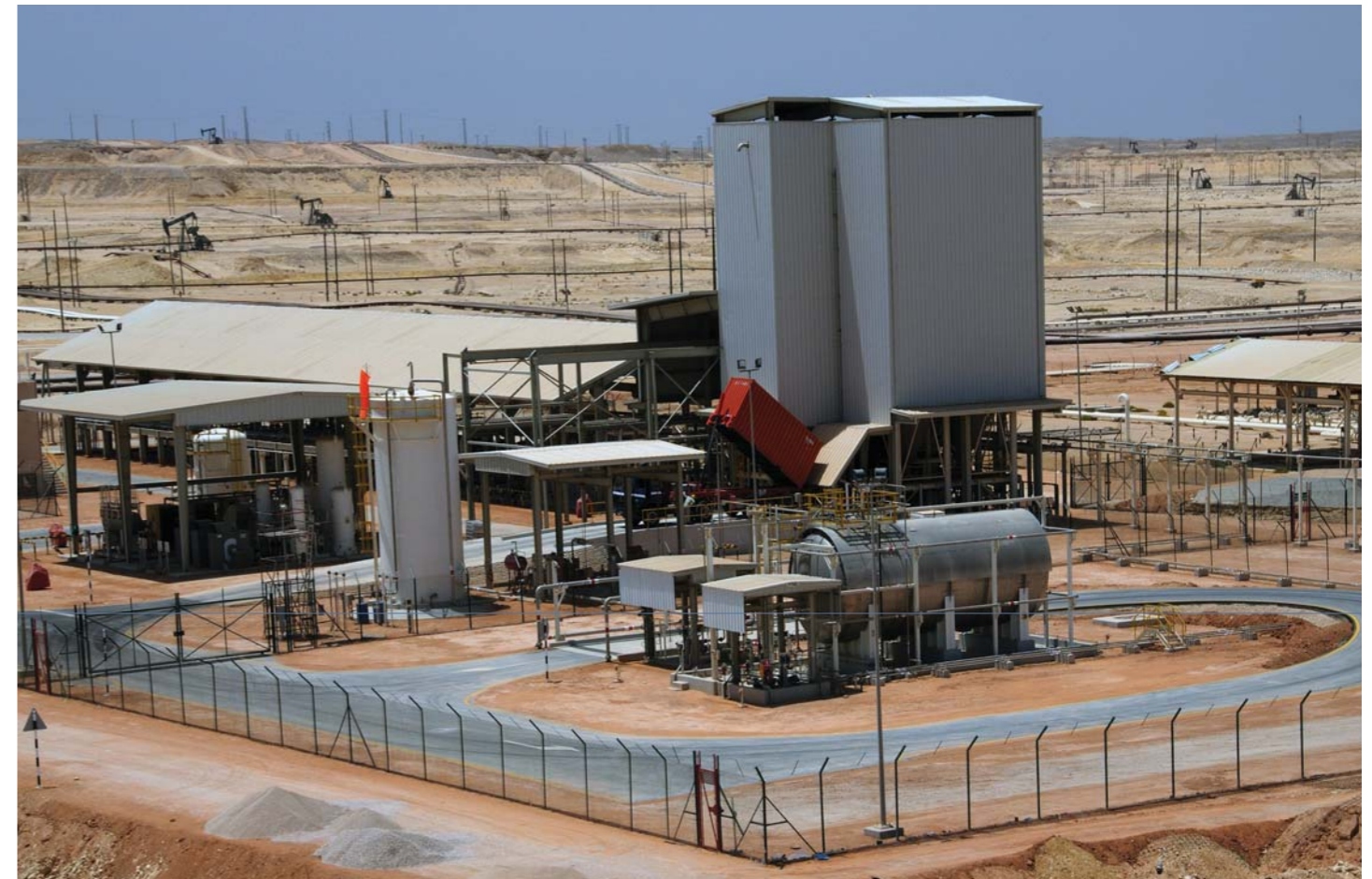
Polymer Storage, Mixing and Injection Facility
