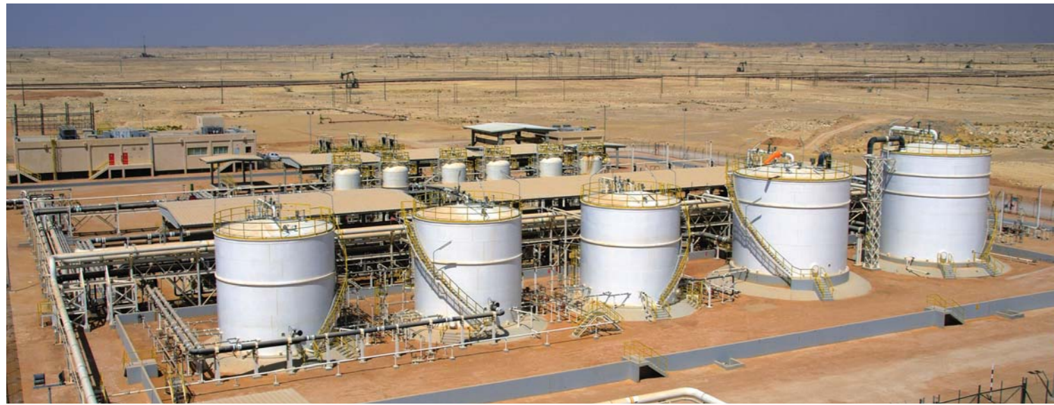
Storage Tanks area in WTP
