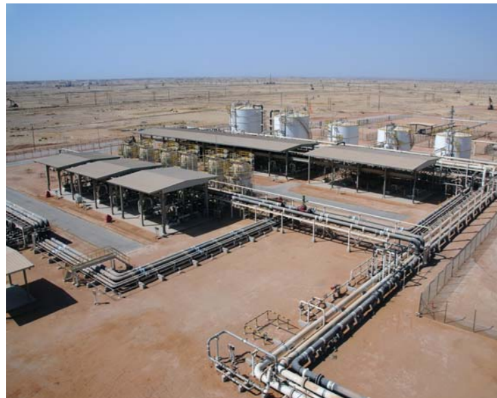
On-plot GRE Piping
