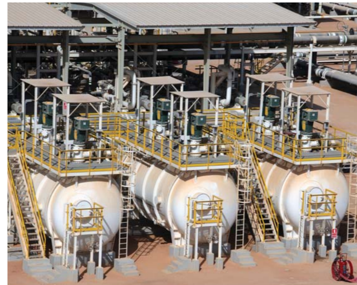
Primary Water Treatment (HDBF) Facility
