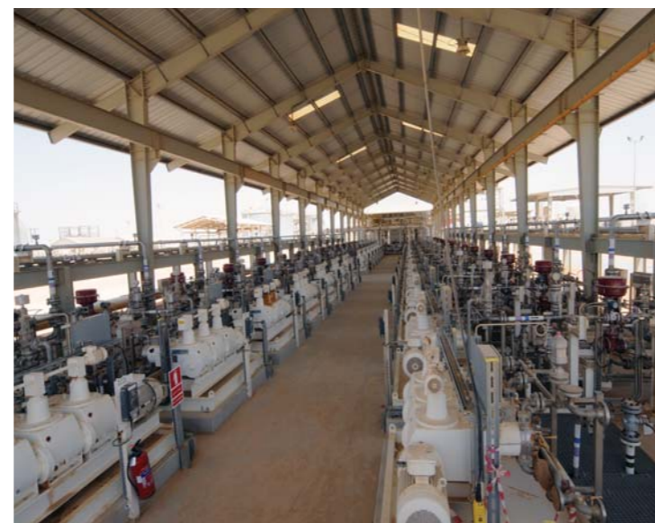
Polymer Injection Pump Bay
