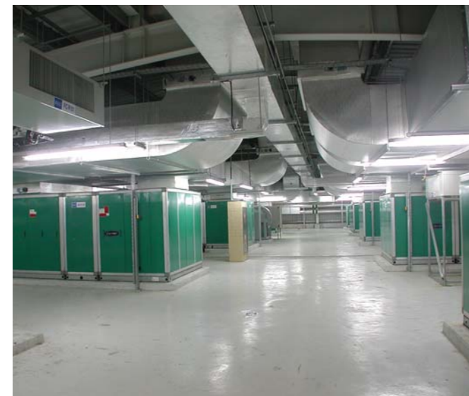
Air Handling Units
