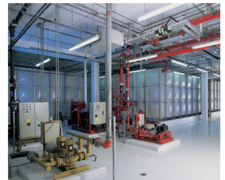
Cold Water and Fire Fighting Pumps
