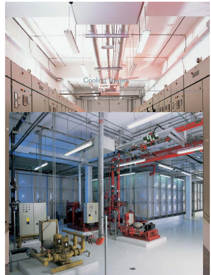
Air Handling Units
