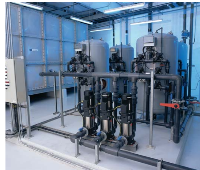
Water Softner Plant
