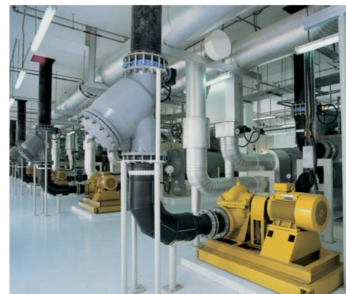
Condenser Water Pumps
