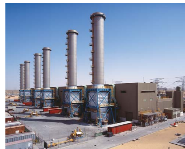
Mechanical, Electrical & Instrumentation construction for 600 MW Al Aweer Power Project including 6X100MW GTG.
