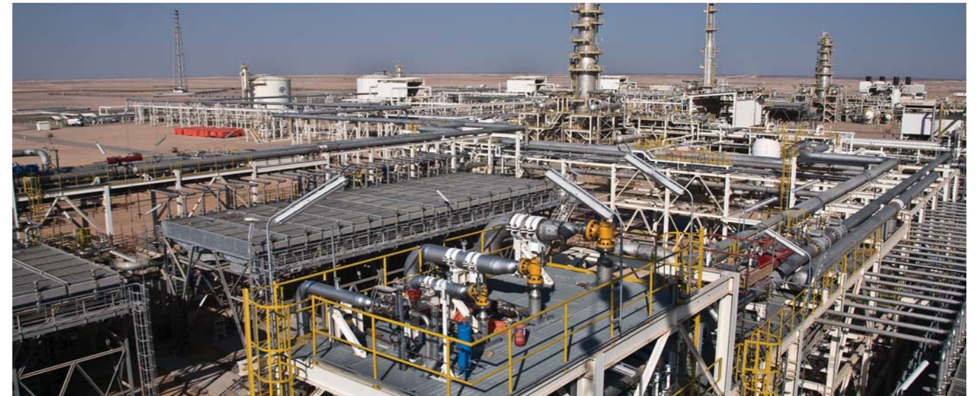
Complete Civil, Mechanical, Electrical & Instrumentation construction for Saih Rawl Depletion Compression Project consisting of 4X30 MW Depletion Compressors, 1X120 MW Power Plant and 132kV/33kV Overhead Line.
