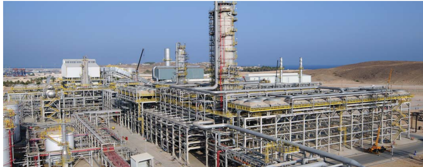
Civil, Mechanical, Equipment Installation and Piping Works for Salalah Methanol Project Process Train.
