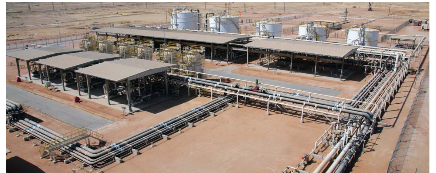
Complete Civil, Mechanical, Electrical & Instrumentation construction for PDO Marmul Polymer Flooding Project - EOR consisting of Water Treatment Plant, Polymer preparation & Injection plant and Flow/Pipelines for 27 Well Heads.
