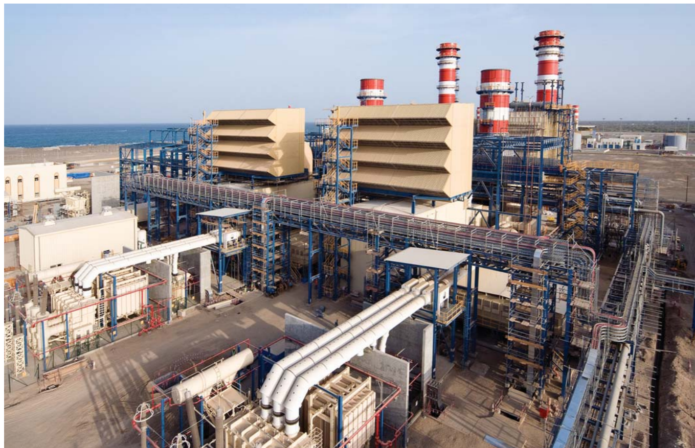
Mechanical, Structural & Piping Installation works for 750 MW Sohar IPP Phase-2 including 2X250 MW GTG, 1X250 MW STG and 2 HRSGs.
