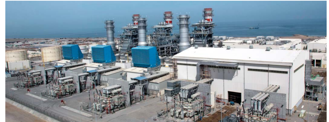
Mechanical, Structural & Piping Installation works for 680 MW Power & 26 MIGD Desalination, Barkha IWPP Phase-2 including 3 X 122MW GTG, 3 X 325T HRSG, 2 X 157MW STG and 26 MIGD RO Plant.
