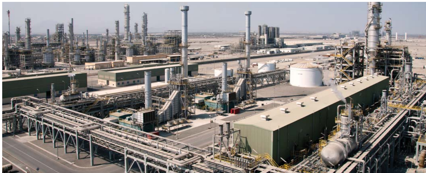
Mechanical, Electrical & Instrumentation works for Fertilizer Plant consisting of 2000 TPD Ammonia and 2X1750 TPD Urea Plants at Sohar.
