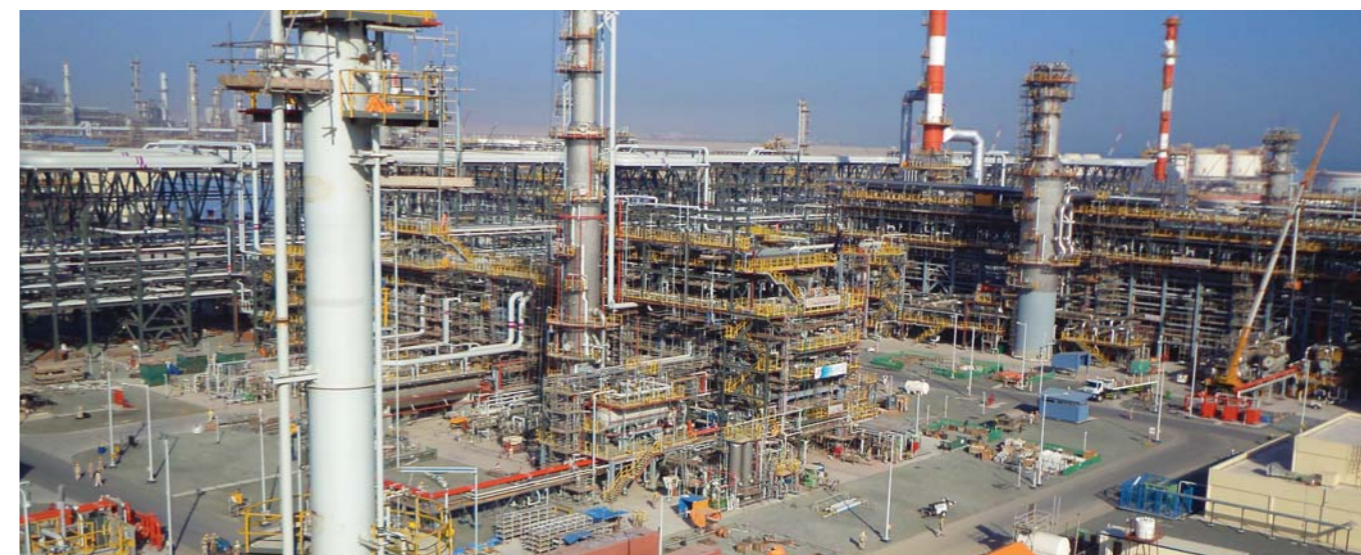
Project Management, Supervision and Mechanical, Structural & Piping Installation works for Ruwais Refinery Project, Abu Dhabi.
