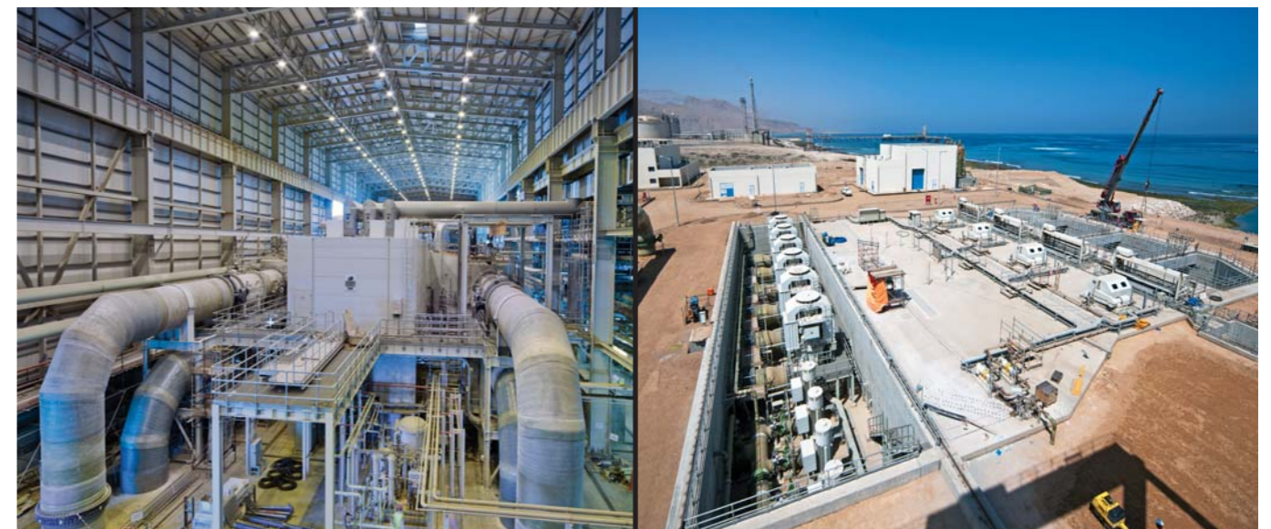
Project Management, Supervision and Mechanical, Structural & Piping Installation works of 3X250 MW STG, Seawater Intake and associated auxiliaries for 2000MW SUR Independent Power Plant.
