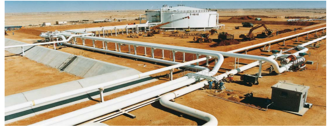
EPC of Free Water Knockout Tank, pumps and related piping works for PDO at Nimr
