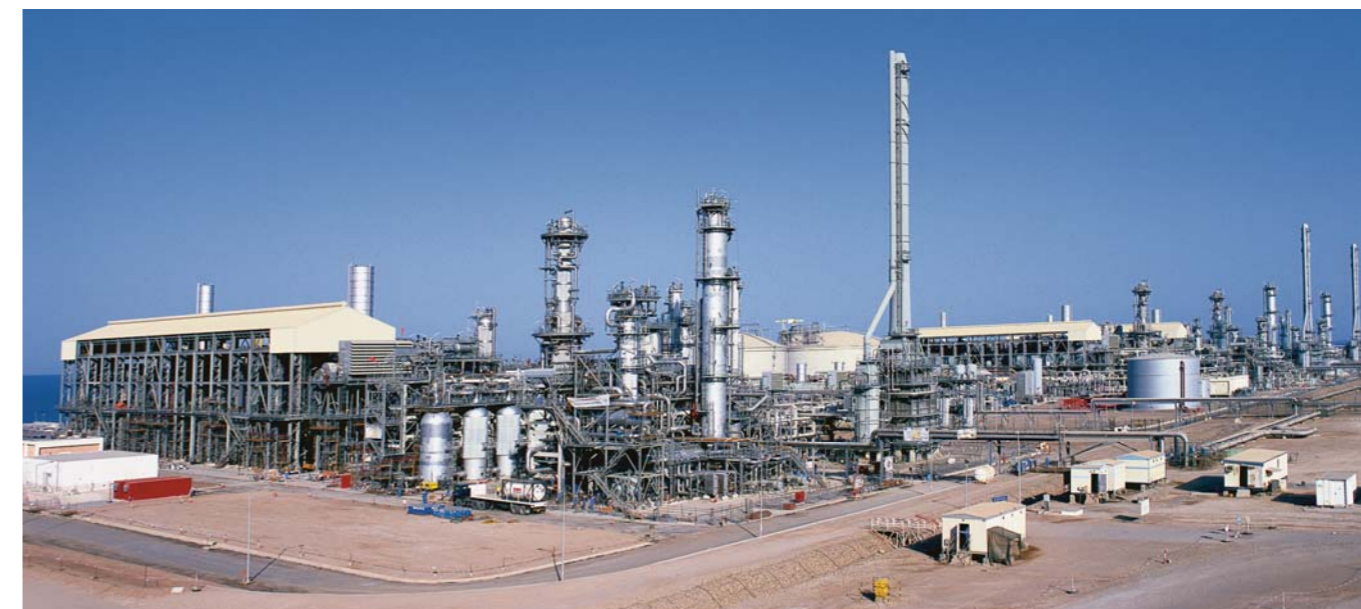
Project Management, Supervision and Mechanical, Electrical & Instrumentation Installation of process works for Qalhat LNG Project.
