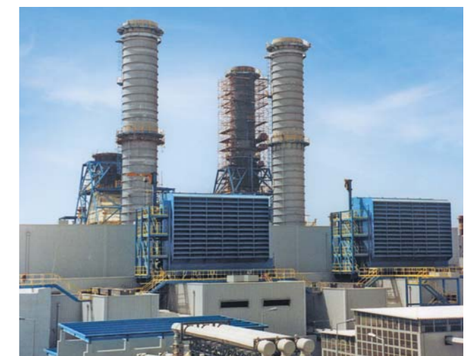
Mechanical, Electrical & Instrumentation works for 450 MW Power Plant at Jebel Ali including 3X150MW GTG.
