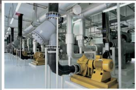
Condenser Water Pumps
