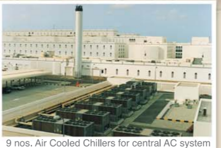
9 nos. Air Cooled Chillers for central AC system
