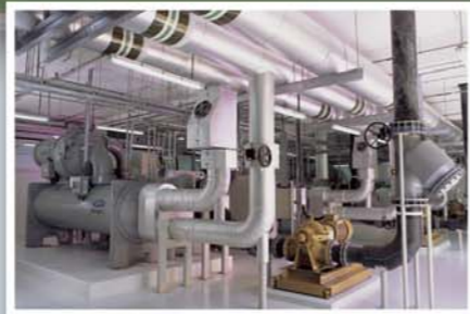
Centrifugal Chillers & Condenser Water Pumps
