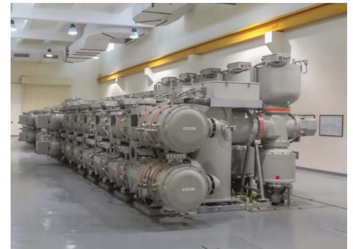
132kV Gas Insulated Switchgear with LCC Panels at Mahadha 132kV Grid Station.
