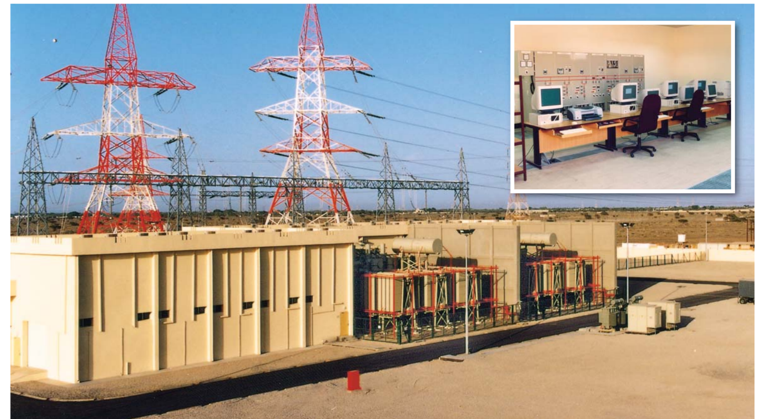
220 kV Sub-station at Felaj for Barka Transmission System with Substation Control System.
