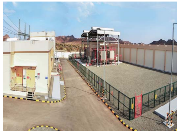
Ibra 132/33kV Grid Station with 2x125 MVA Transformers
