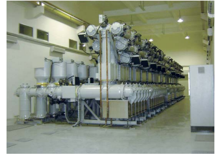
220 kV GIS at Sohar Power Station Sub-station
