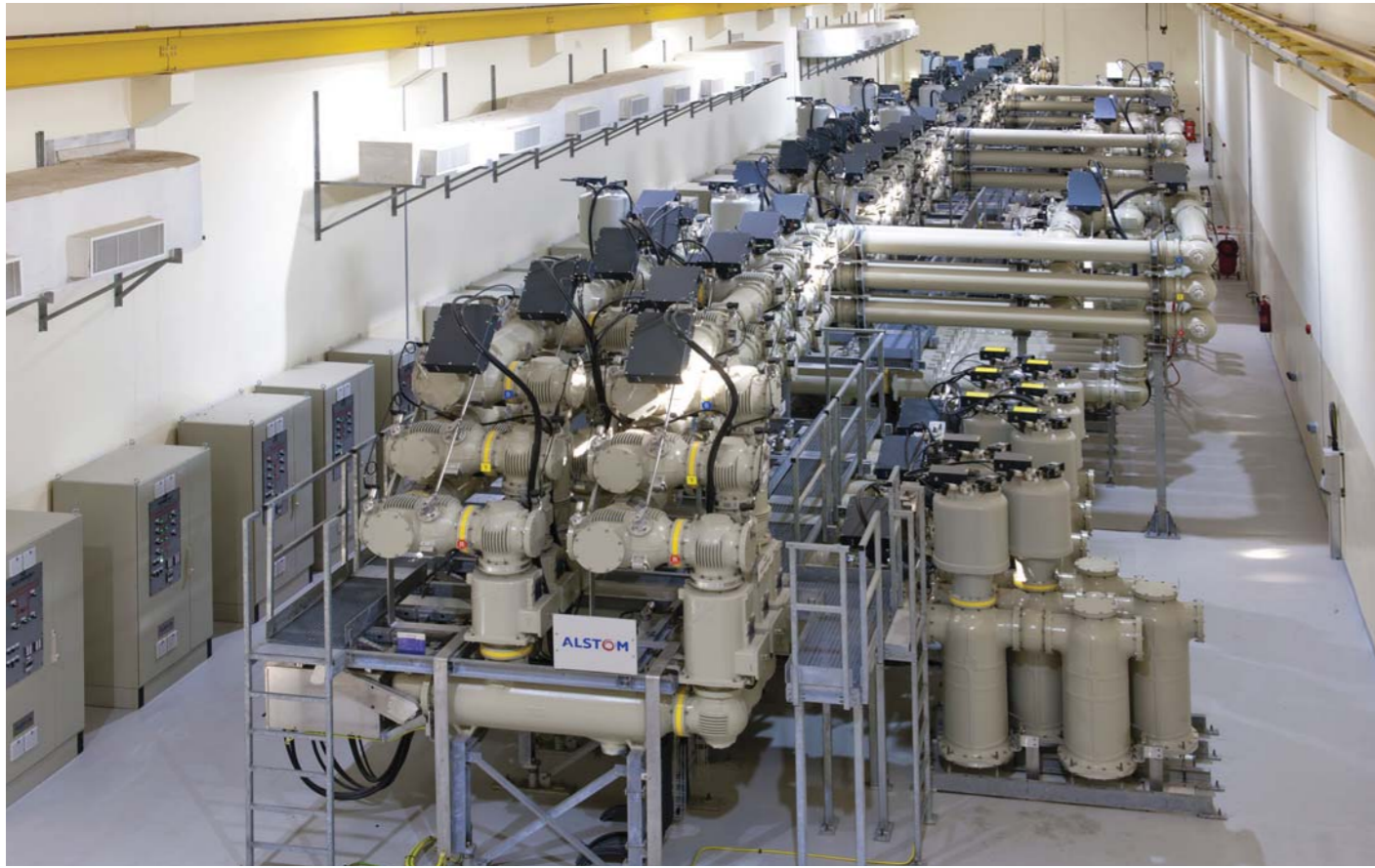
220 kV Grid Station at Sur, the largest in Oman, for Oman Electricity Transmission Company.
