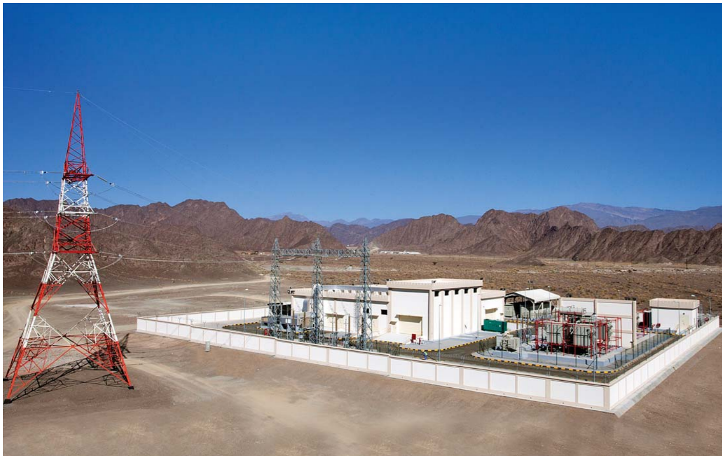
132/33 kV Grid Station - Madinat Nizwa
