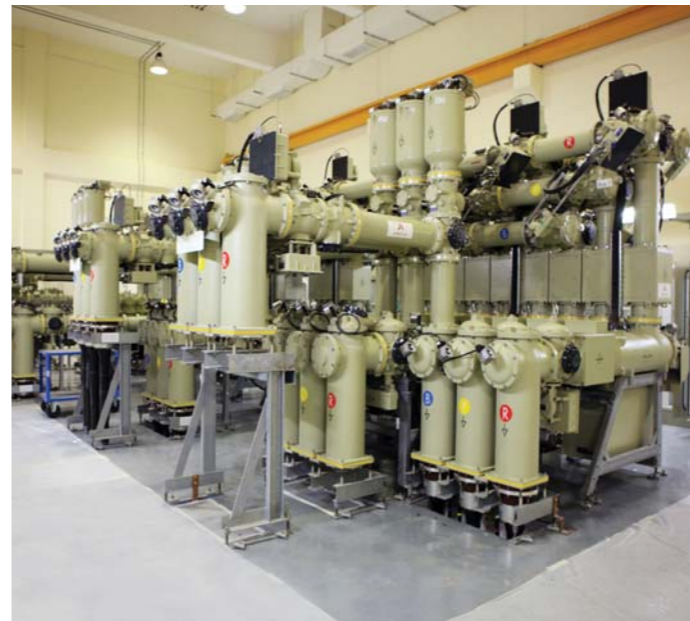
132 kV GIS at Al Quoz substation - DEWA
