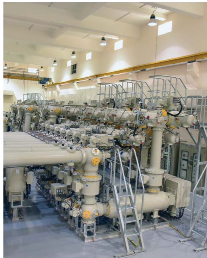
220kV Gas Insulated Switchgear at Mabella-1 Grid Station
