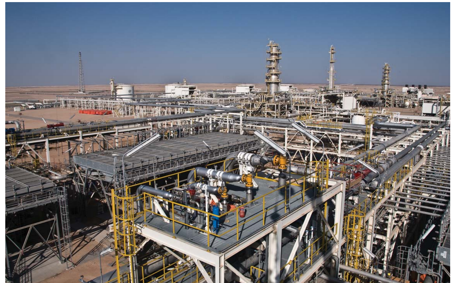
A view from the Pipe Rack
