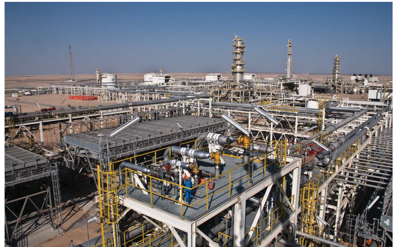
A view from the Pipe Rack
